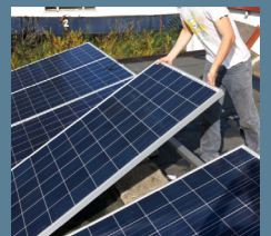
Generate a local smart grid for the efficient usage of solar energy Source: Deceuvell
